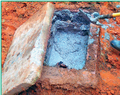
Corroded Concrete Interceptor Typical life expectancy is 10 years.
