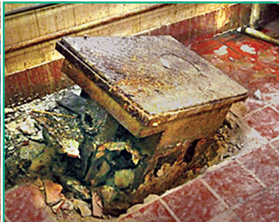
Rusted Steel Grease Interceptor Typical life expectancy is 5 years.
